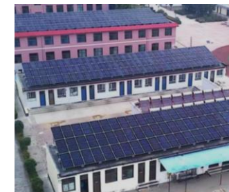
Solar rooftop at school site
