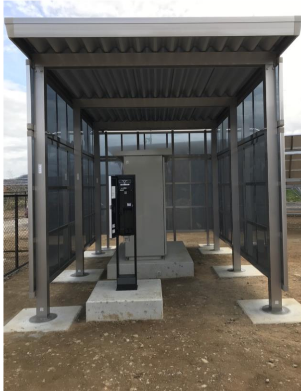
The emergency power supply system at Nari Aizu Solar Power Plant provides charging services to city residents during a power outage.
